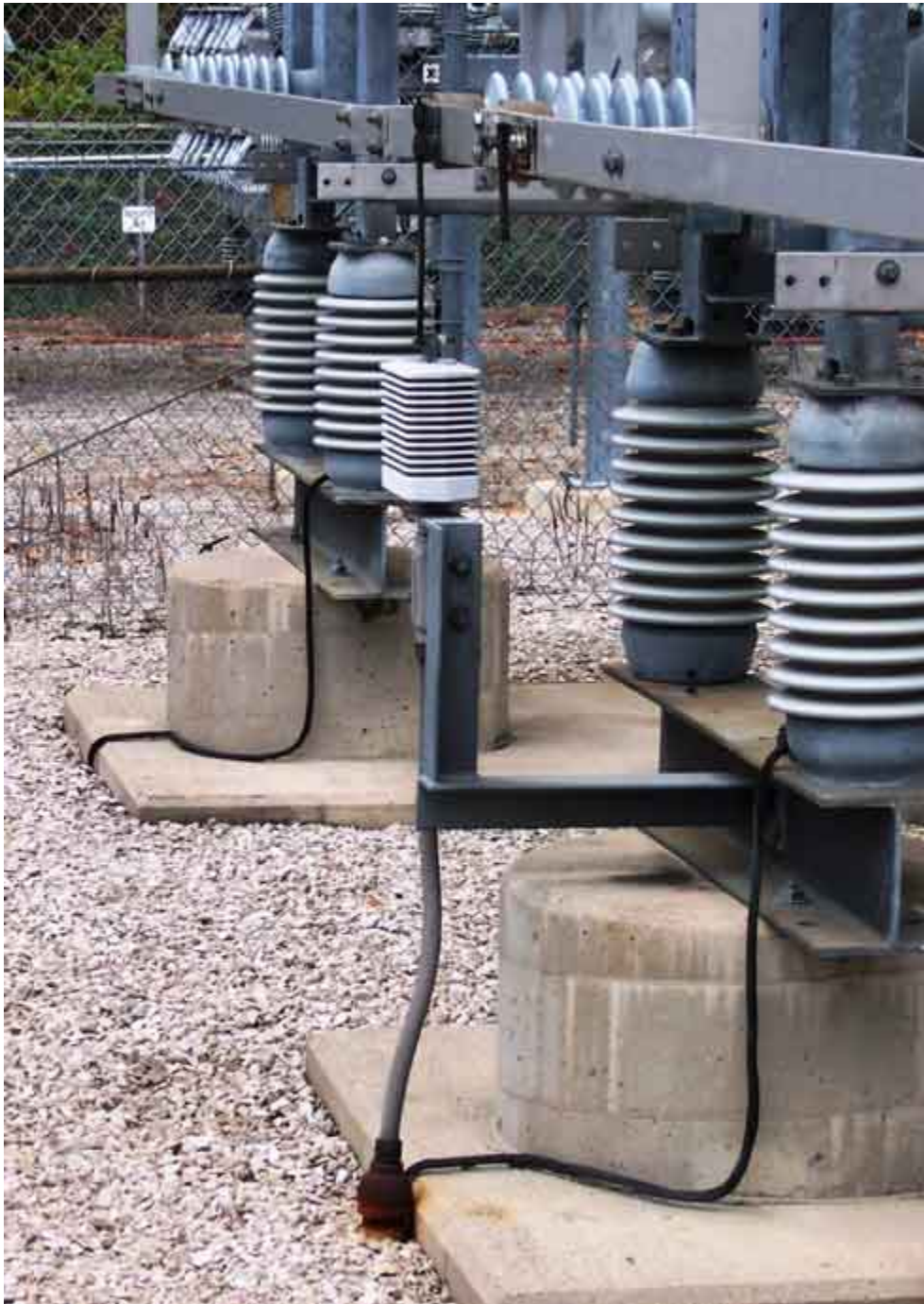
Figure 05 — Voltage-Sensing Potential Device
